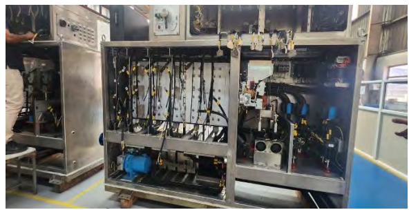
Traction Converter (under assembling process)
