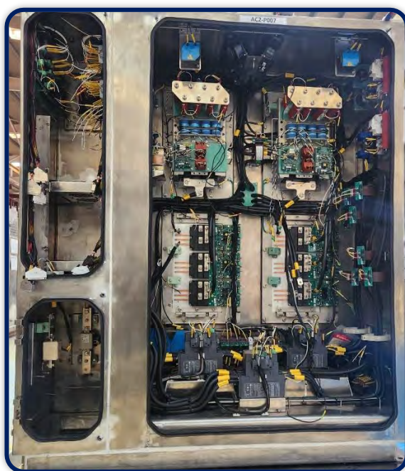
Inside view of Auxiliary converter
