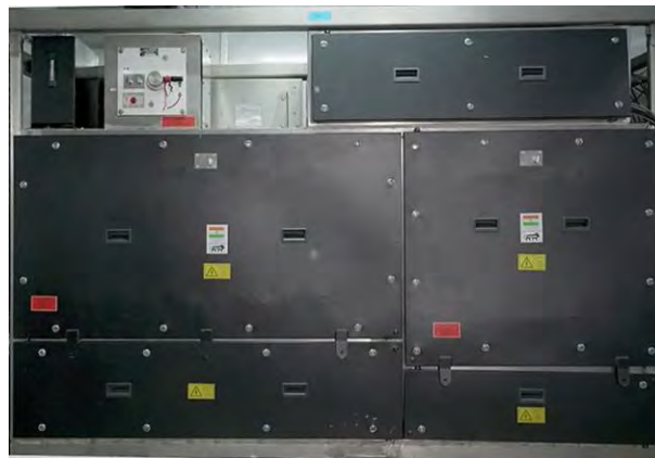
Outside view of traction converter
