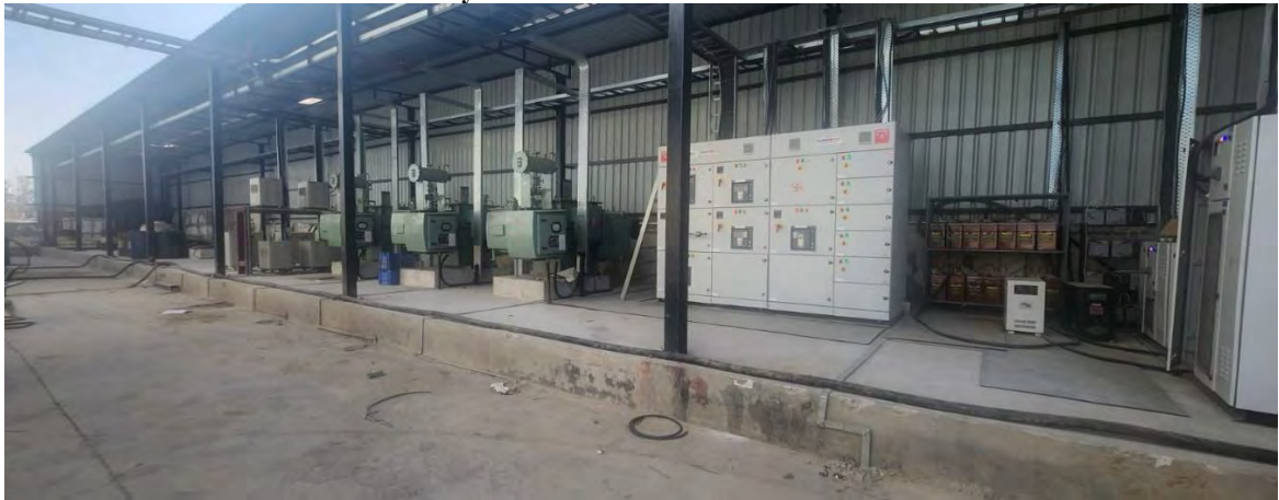
Transformers for Test Set up
